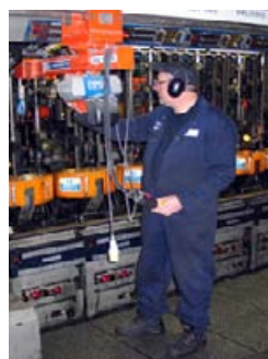
Figure 4: Fixed Lifting Equipment
